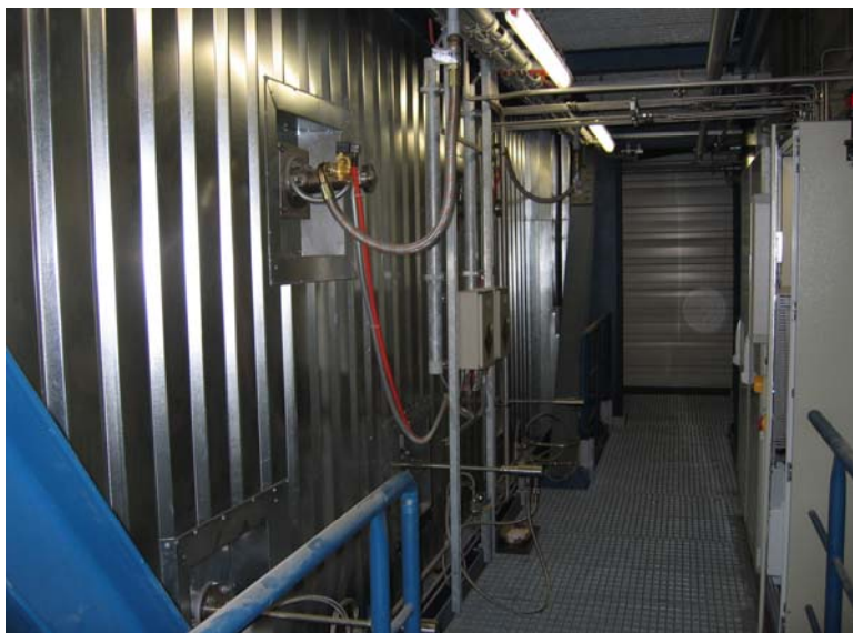
Pic 6: SNCR Injection Lances with Acoustic Temperature Measurement (agam)
