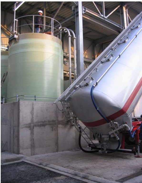
Pic 4: Mixing Station and Storage Tank for Urea Solution
