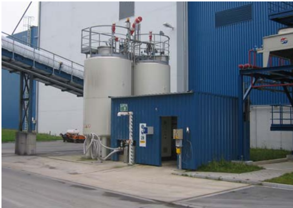
Pic1: Storage Tank for Ammonia Water with Pumping Station
