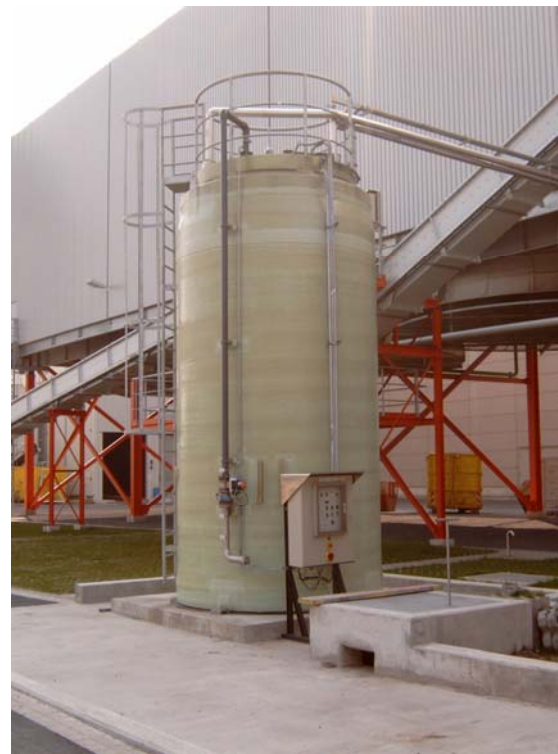
Pic 5: Storage Tank for Urea Solution
